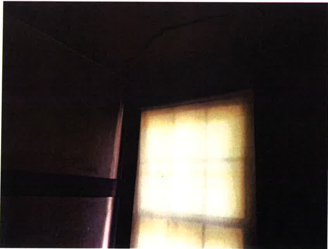
Cracks throughout interior ceiling
