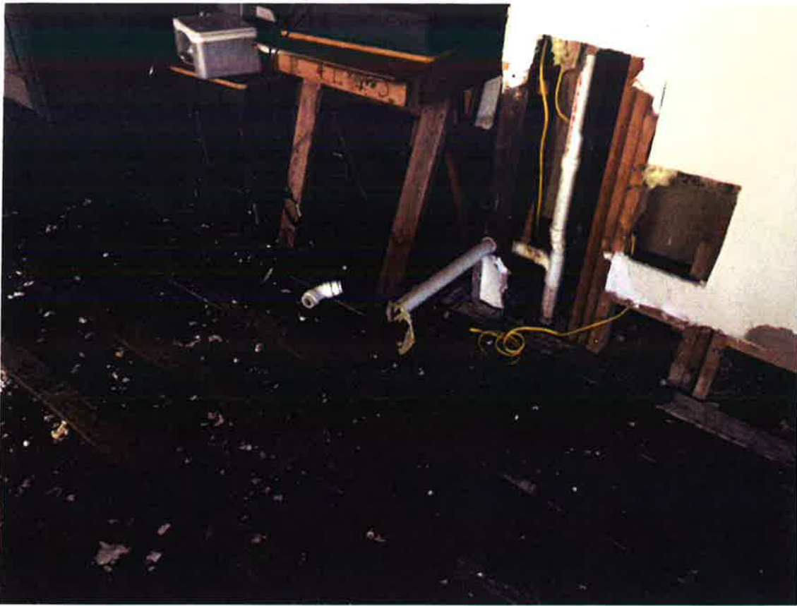
Interior fixtures and appurtenances have been removed. Extensive water damage with mold throughout structure.
