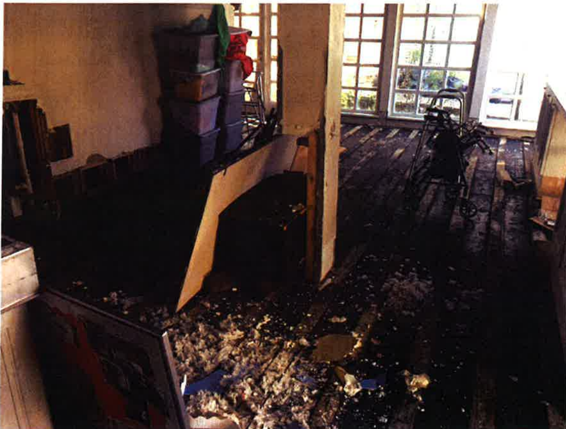
Interior fixtures and appurtenances have been removed. Extensive water damage with mold throughout structure.
