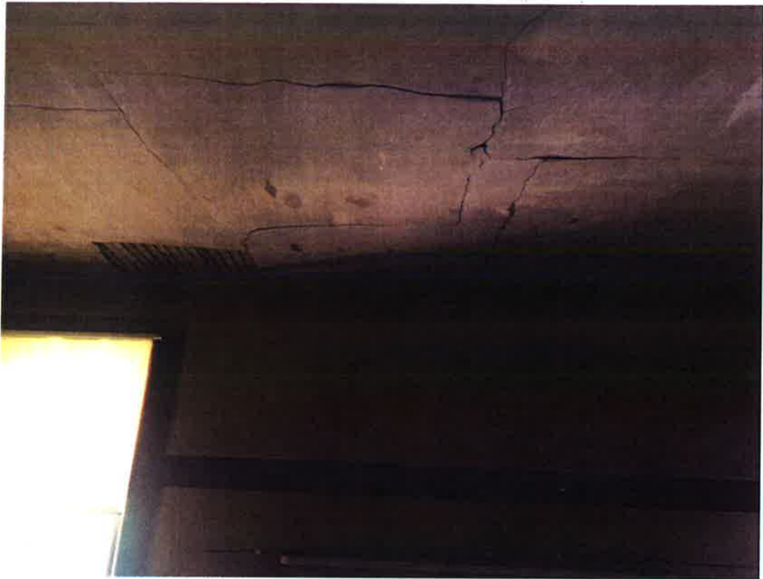
Cracks throughout interior ceiling
