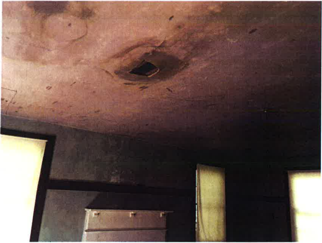
Cracks throughout interior ceiling
