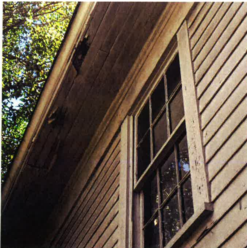
Wooden eaves are rotten
