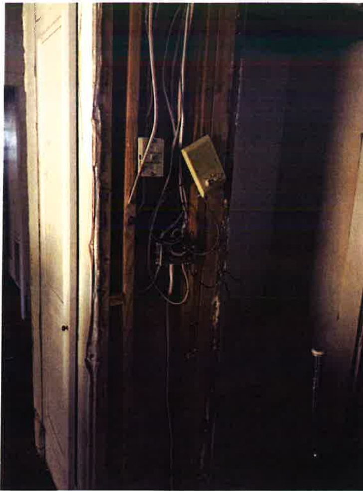
Interior fixtures and appurtenances have been removed. Extensive water damage with mold throughout structure.
