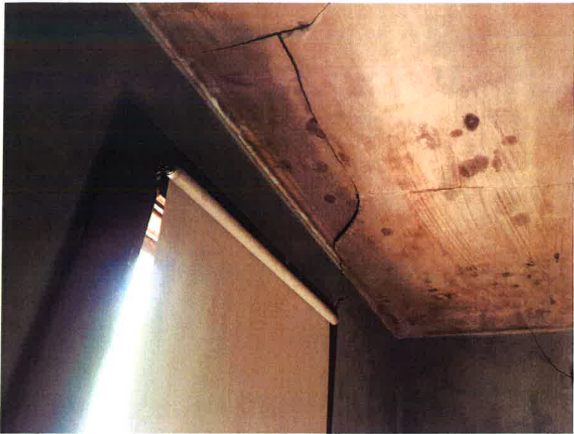
Cracks in interior walls and ceilings caused by shifting
