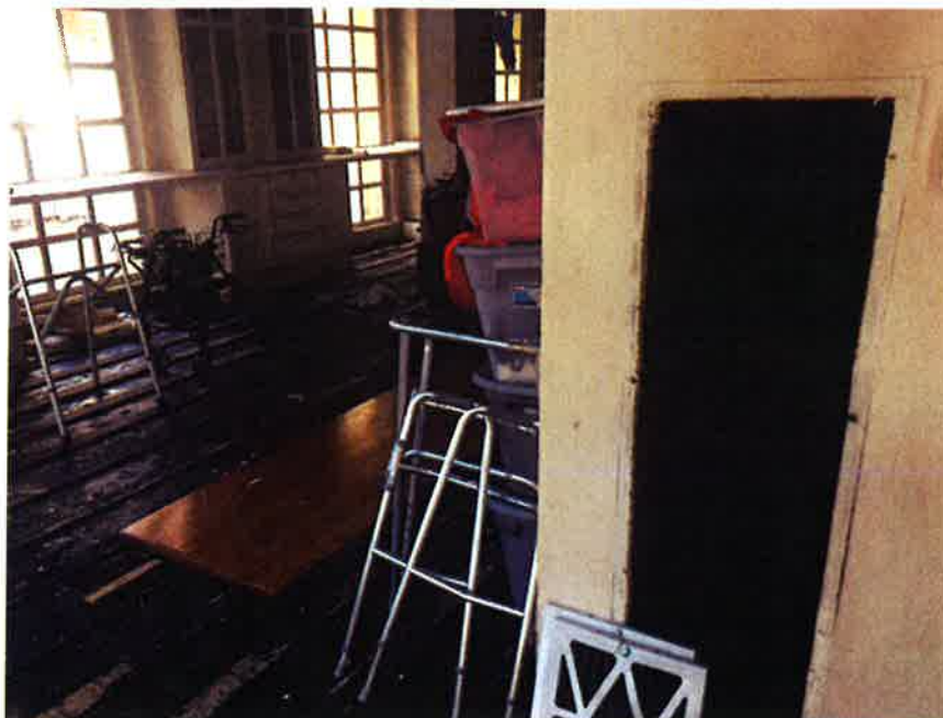
Interior fixtures and appurtenances have been removed. Extensive water damage with mold throughout structure.
