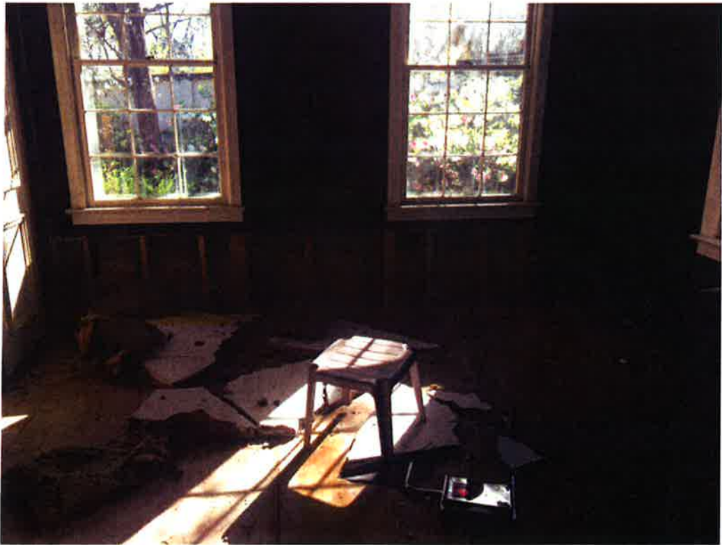
Extensive water damage with mold throughout structure
