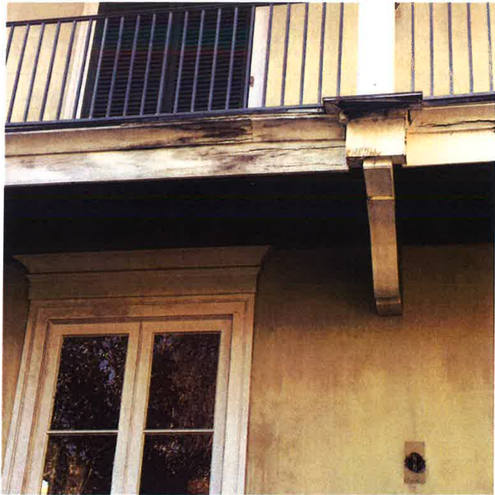
Rotten wood on exterior of structure
