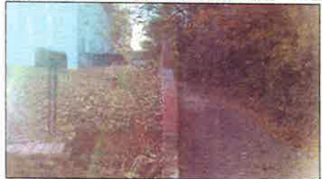
WALL IS FAILING; WALL TO BE LOWERED AND GRADE SLOPED BACK
