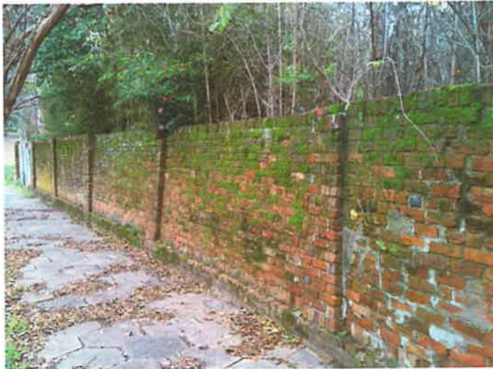
GARDEN WALL (CLANTON ST.)
