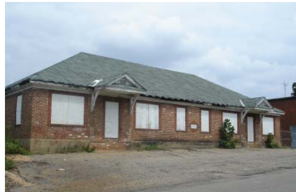
At risk frontage
