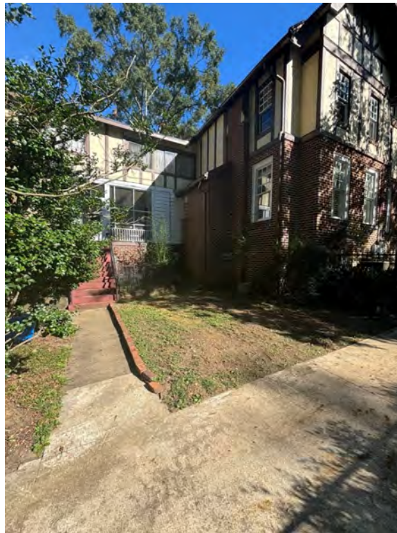
Figure 3c: Existing conditions of the project area (rear inside corner of the home) at 831 Felder Ave.
