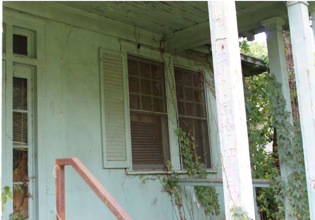
Figure 2b: 620 Ponce de Leon Ave, typical window (in fair condition, at least on the exterior)
