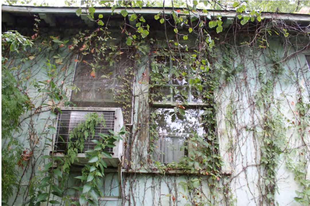
Figure 2c: 620 Ponce de Leon Ave, typical window (in poor condition)
