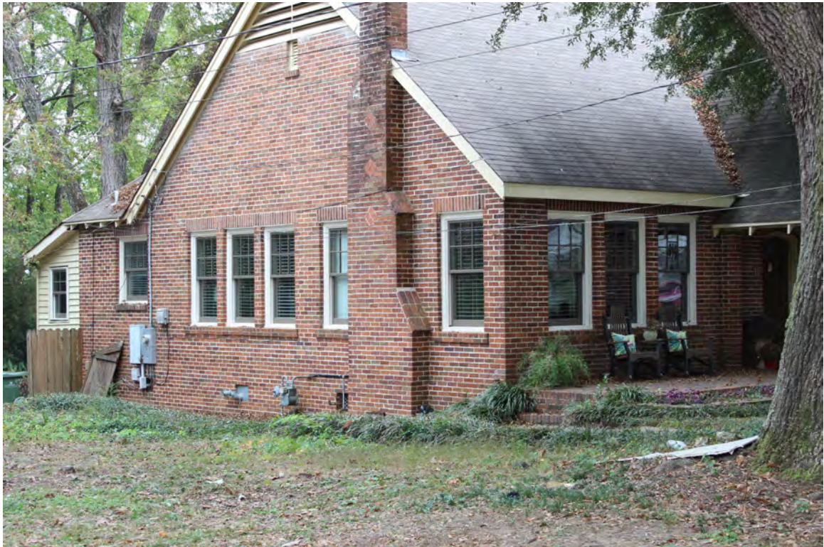
Figure 1k: Example of similar brand and material of windows previously approved by the board at 3143 Lexington Rd.
