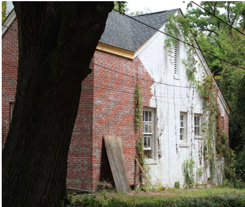
Figure 1h: Location of proposed new window (top right) on the South elevation
