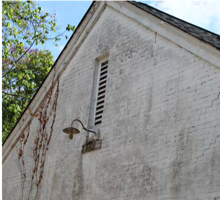
Figure 1i: Detail of existing vent where proposed new window is requested on the North elevation
