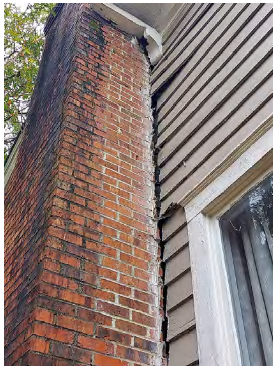
Figure 5d: Detail depicting chimney separating from the wall, 1852 Graham St., 10/22/2024
