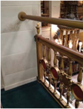
Figure 10. A modern horizontal element was installed to meet the code-required railing height while still retaining the lower historic railing. Photo: Nicholas Vann
