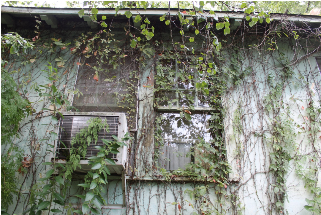
Figure 4c: 620 Ponce de Leon Ave, typical window (in poor condition)
