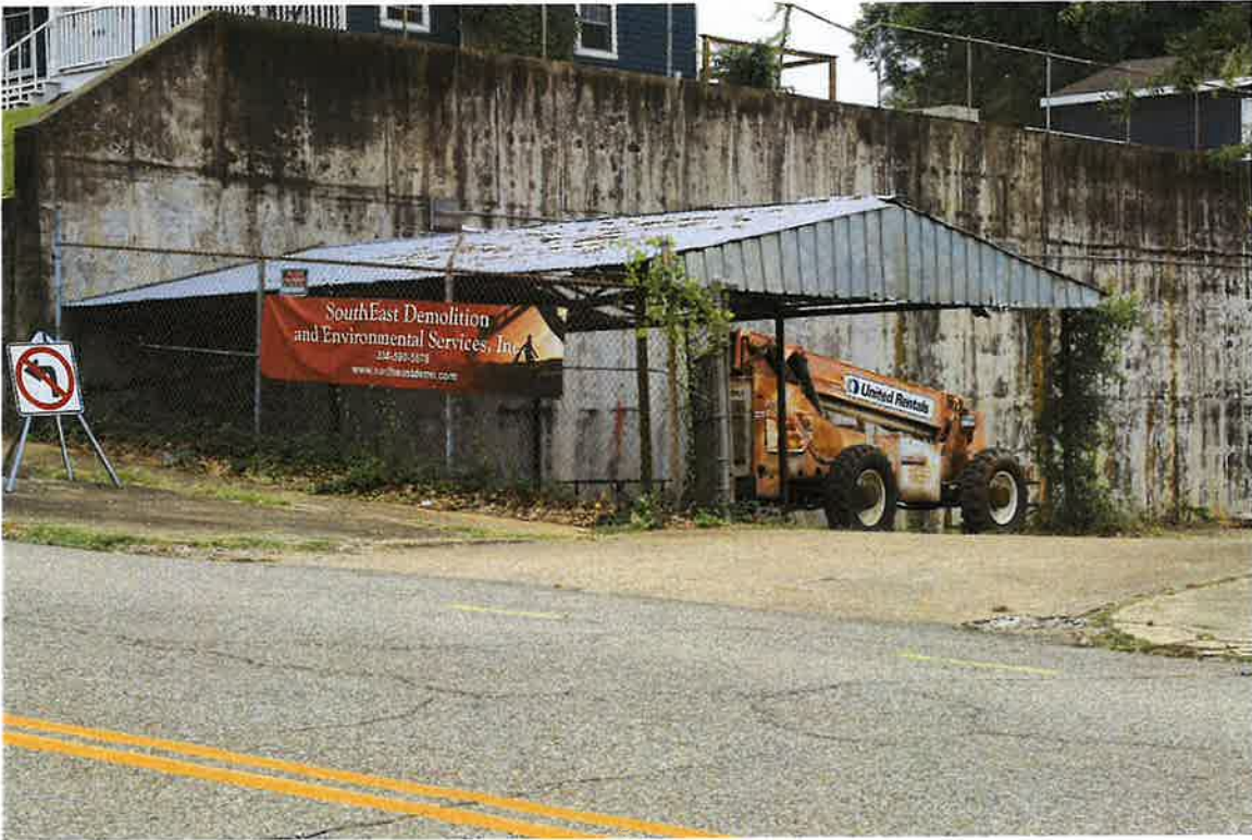
121 N. Goldthwaite Street (Cottage Hill), east elevation within inner courtyard, metal carport, and fencing, 06/05/2024
