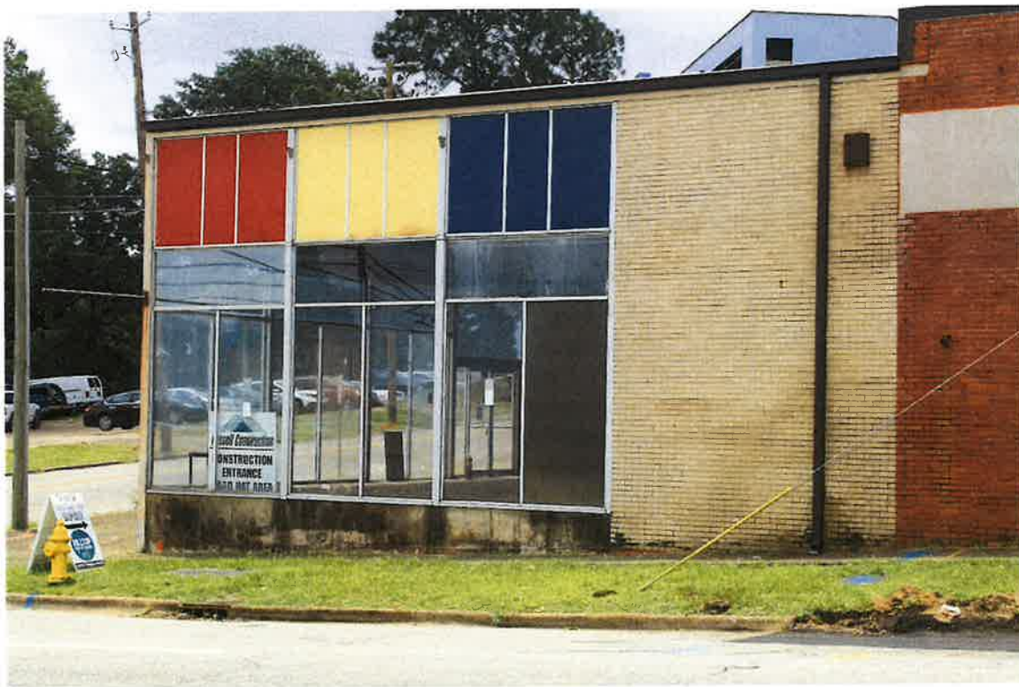
121 N. Goldthwaite Street (Cottage Hill), north elevation and front corner detail from Heron St., 06/05/2024
