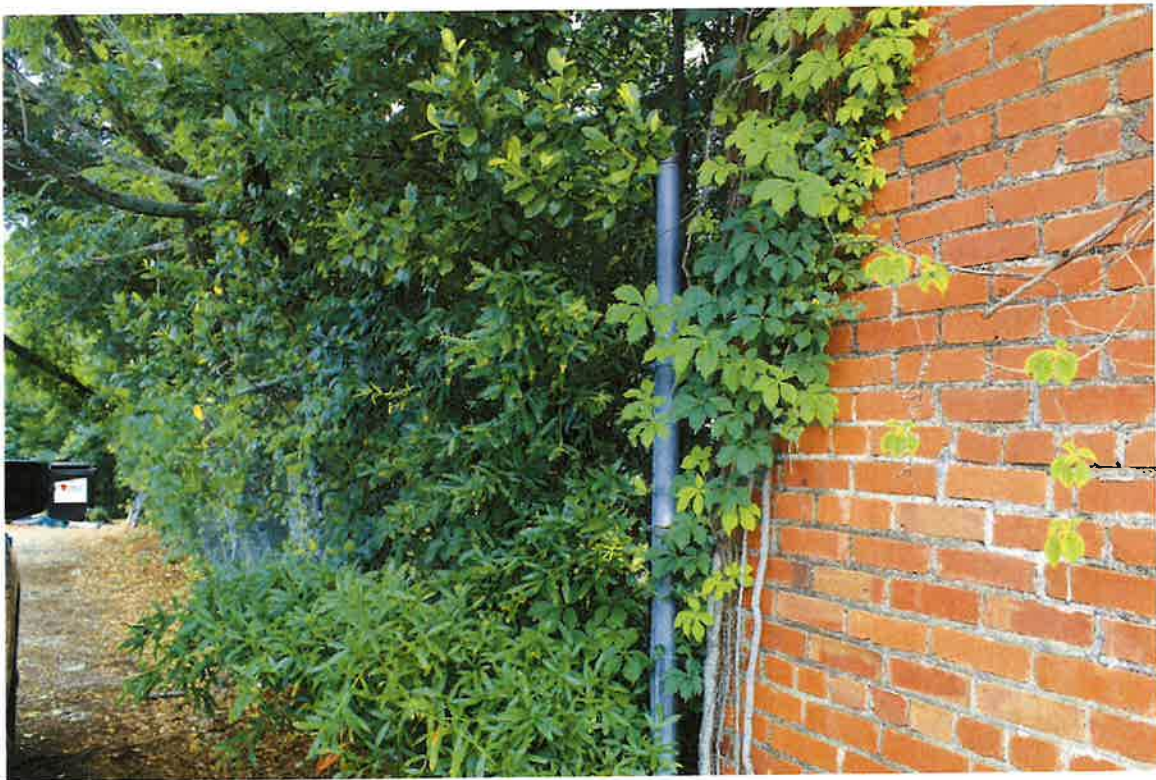
15 N. Goldthwaite Street (Cottage Hill), existing chain link fence along south property boundary and fence detail, 05/10/24
