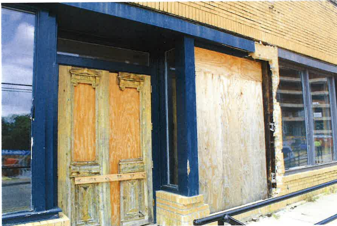
15 N. Goldthwaite Street (Cottage Hill), east façade and deteriorated storefront detail, 05/10/24
