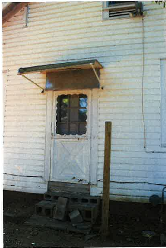
1717 S. Hull Street, detail of western-most door and door in the middle, Garden District, 04/04/24
