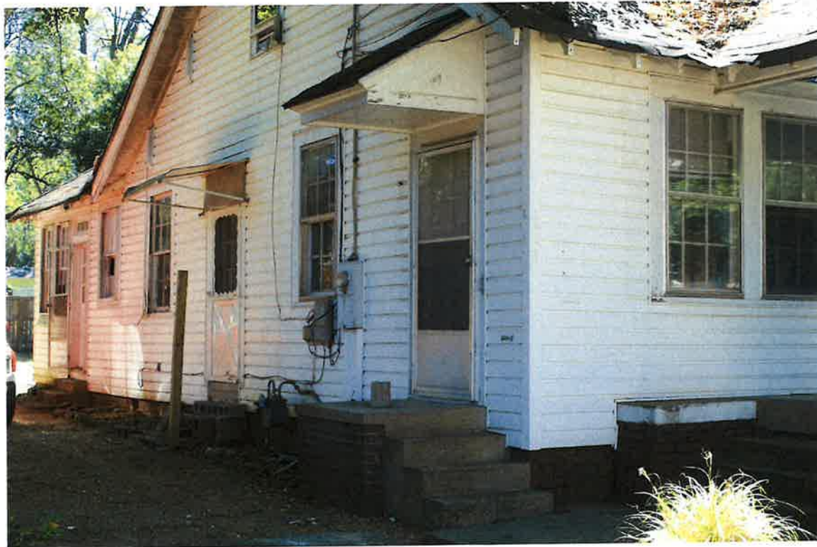
1717 S. Hull Street, Garden District, east façade and three doors to be removed on north elevation, 04/04/24
