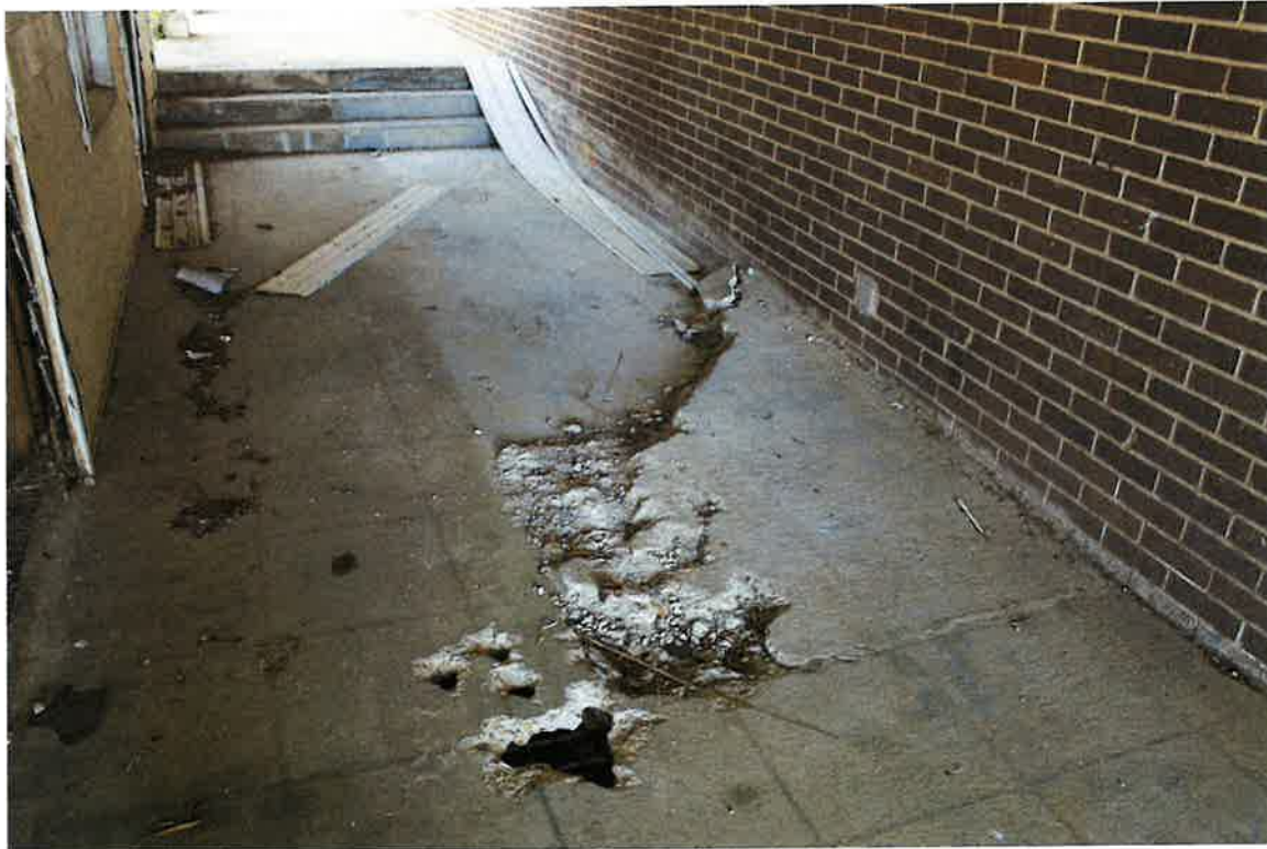
1020 Maxwell Boulevard (Individual Designation), north (rear) elevation and detail of walkway between main building and outbuilding to be demolished and rebuilt in concrete, 04/04/24
