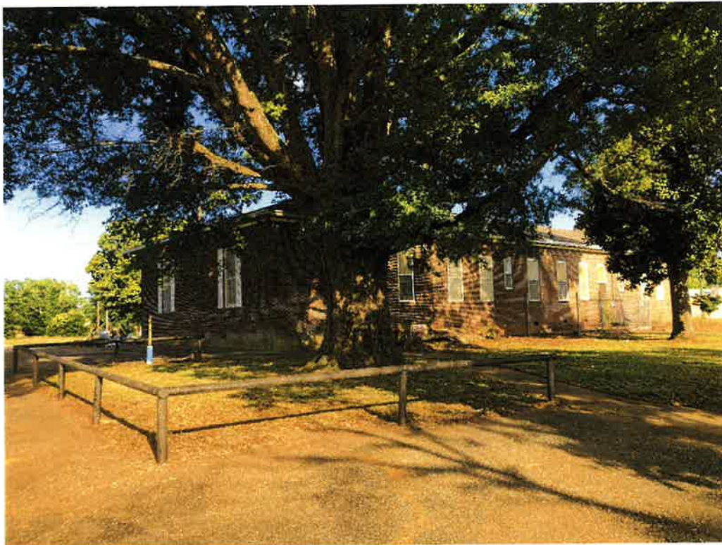
1020 Maxwell Boulevard (Individual Designation), detail of west elevation window to be altered to install an entry door, deck, and egress stairs, and new driveway area at northwest, 04/04/24
