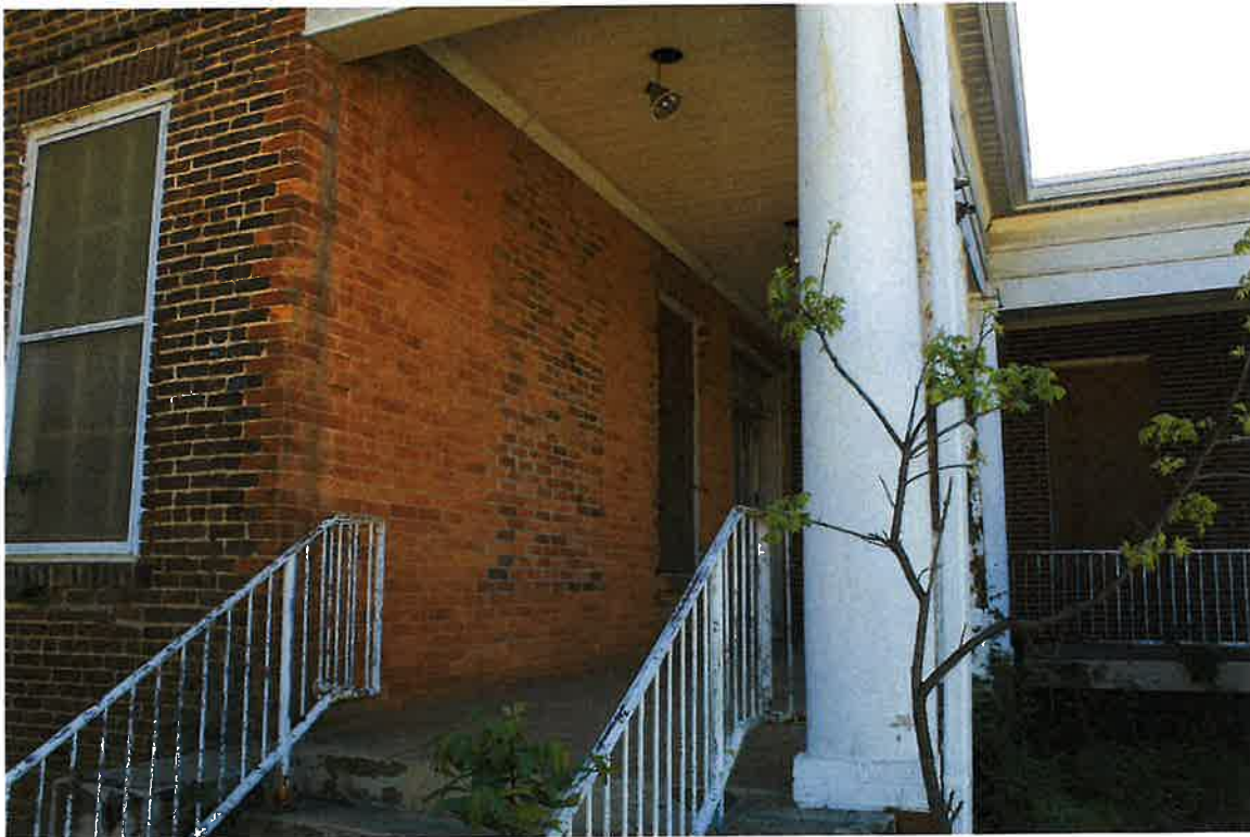
1020 Maxwell Boulevard (Individual Designation), east elevation, looking northwest, and detail of historic brick replacement or alteration, 04/04/24
