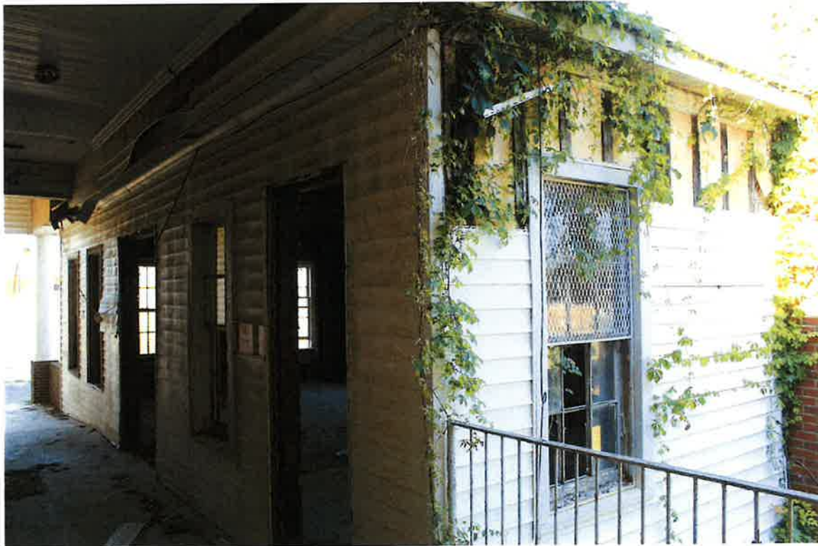
1020 Maxwell Boulevard (Individual Designation), detail of entry door to be repaired or replaced, and west elevation of the added outbuilding, 04/04/24
