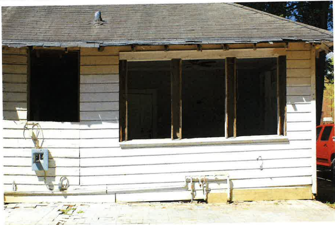
1717 S. Hull Street, east (rear) elevation and detail of rough window openings, Garden District, 04/04/24
