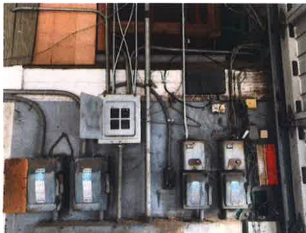
ANTIQUATED ELECTRICAL SYSTEM
