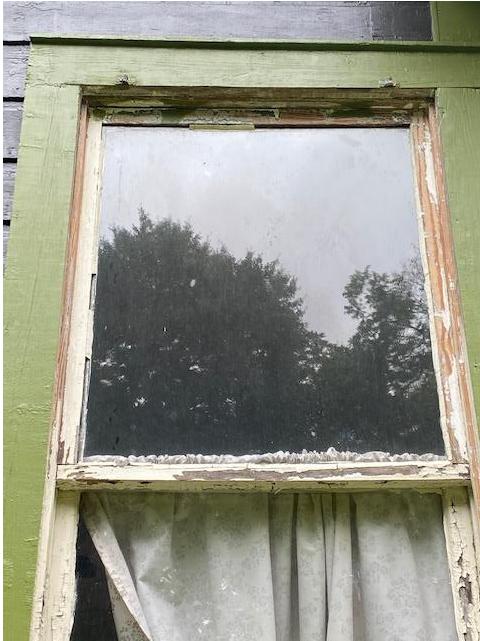
Glazing is missing, paint failing
