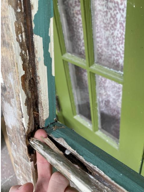
Rot in muntin and stile due to water
