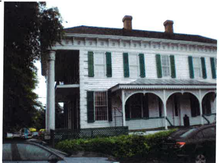
East side with metal porch roof to be replaced with like material
