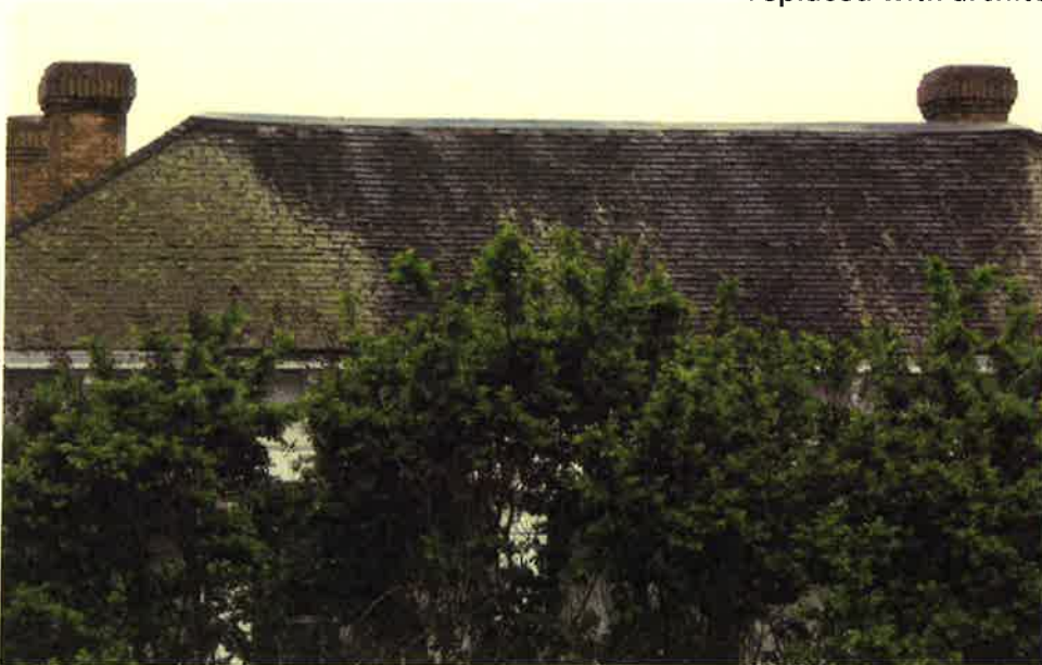
Overall condition with view of flat top to be replaced with insulation and membrane
