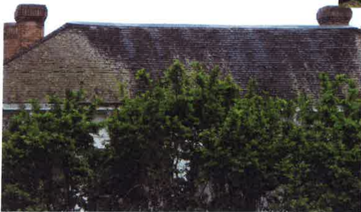
Overall condition with view of flat top of tar and paper to be replaced with like material
