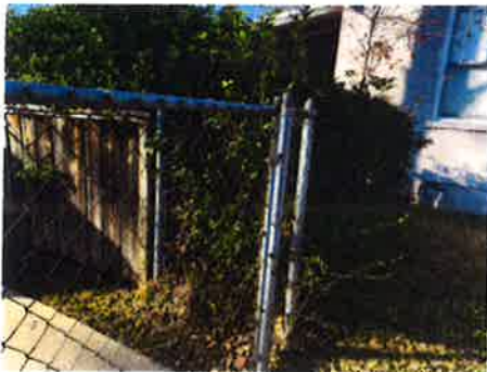
Chain-link fence and posts to be replaced
