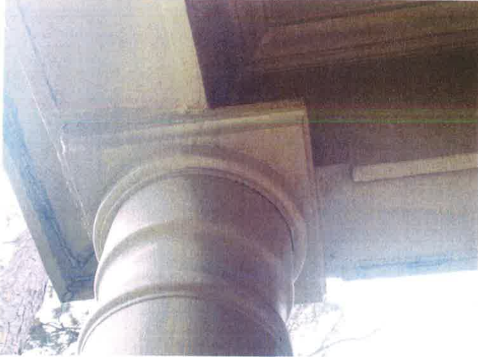
5. Disruption to original woodwork at the top of the front left column.
