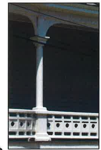
ARCHITECTURAL DECORATIVE DETAILS PHOTO OF DETAILS TO MATCH RELATED TO THE COLUMNS AND UPPER COLUMN CORNICE. THE PICKETS WILL BE AS NOTED ON THE ELEVATIONS
