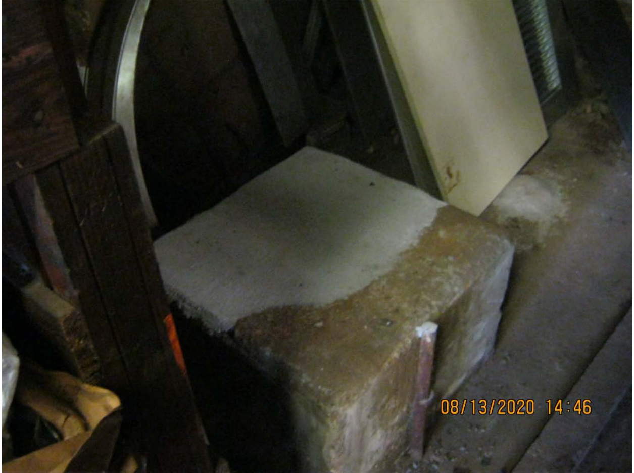
520 North Court Street - Abandoned Bus Washing Well
