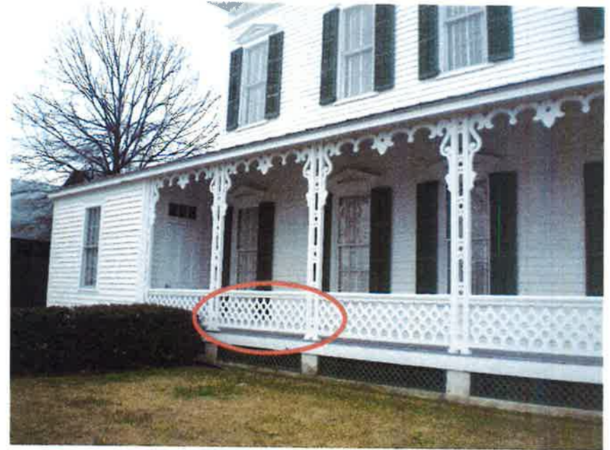
North side, wooden step installation with simple iron handrails on either end
