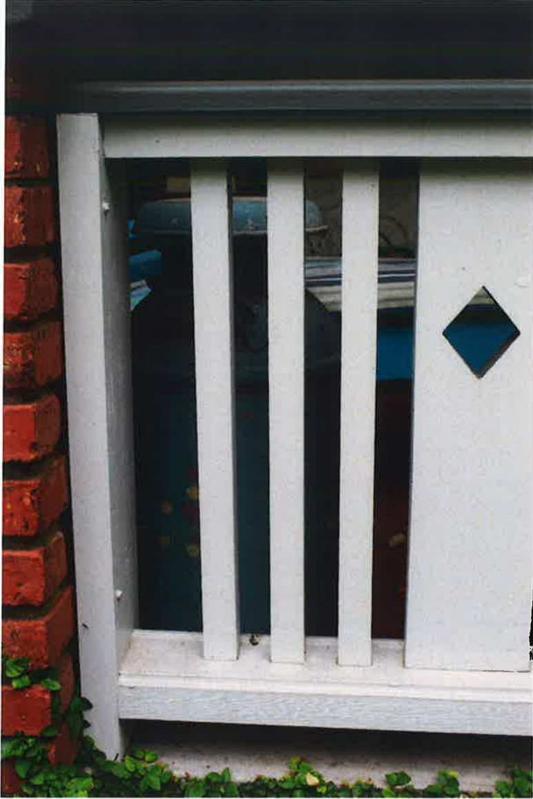
Porch rail example, balusters and rail system only (not the diamond panel)
