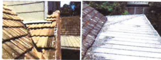
*Some of the roofing tiles are damaged. Acceptable
