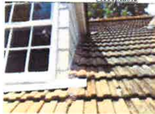
FYI: The sidewall flashings have been sealed with cement, which must be maintained to prevent leaks.
