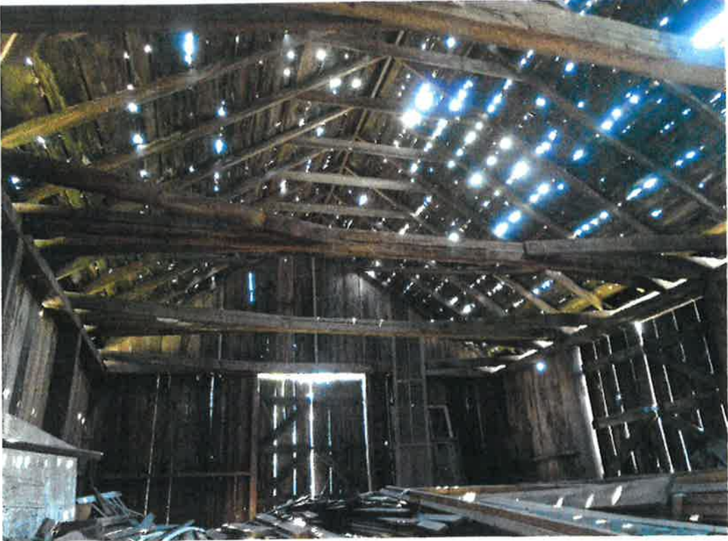
Interior view of damage
