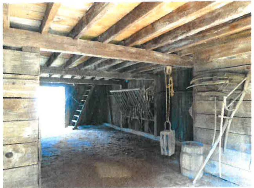
Interior view, water damage
