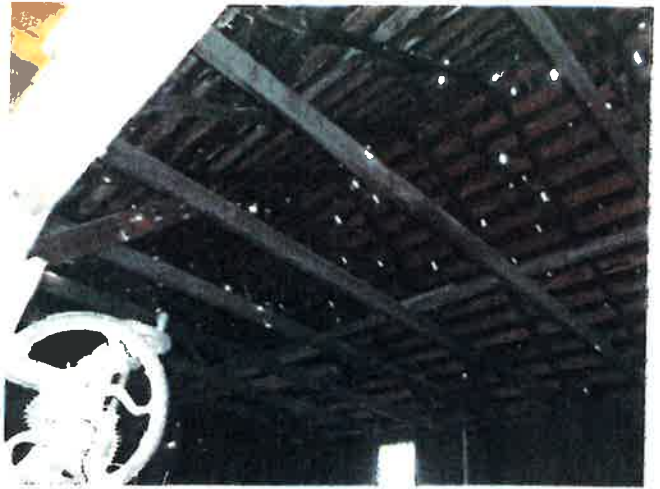
Interior roof damage
