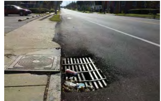
Non-standard drainage grate in the bike lane on Hall Street
